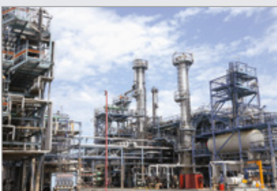
Refinery equipment (option)
